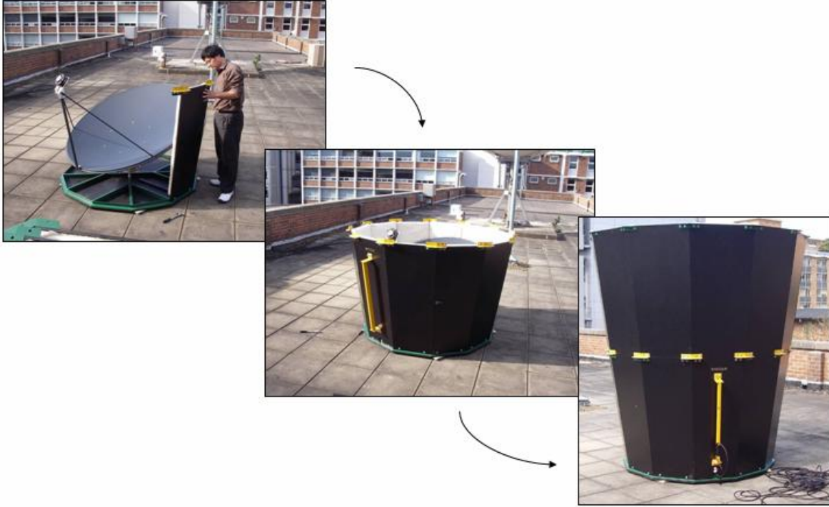
Fig 3 Left: The parabolic reflector mounted on the base plate with the transducer installed at its focus. Middle: First layer of panels installed. Right: The fully constructed sound cone.
